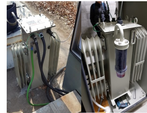
New Generation Transformer Rectifier (新型高频整流变压器)
