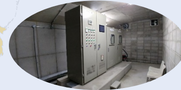
Tunnel Dust Collection
